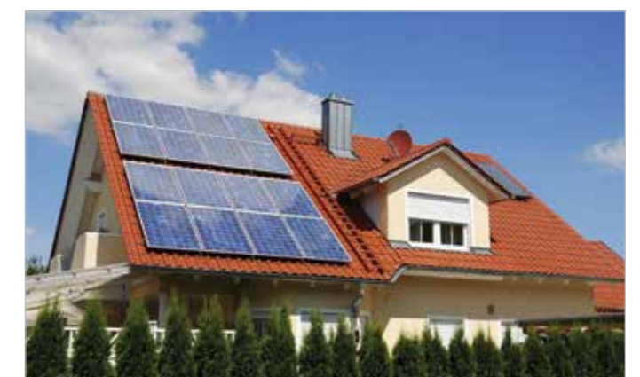
Installations solaires (panneaux)
